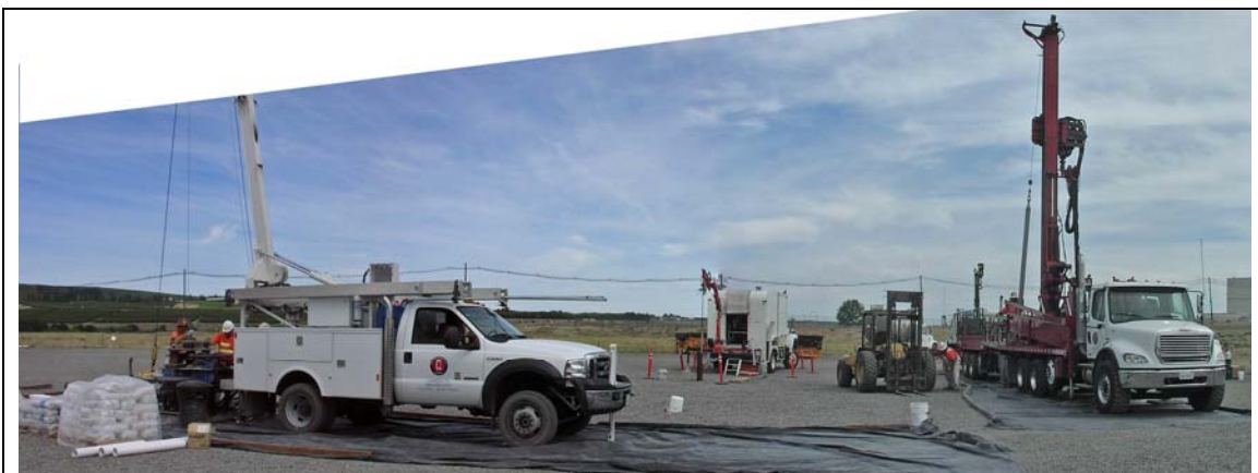
Figure 1. Well drilling at the Hanford IFC site. Resonant sonic rig is on the right, spectral-gamma borehole logging is in the center, and well completion rig is to the left.
