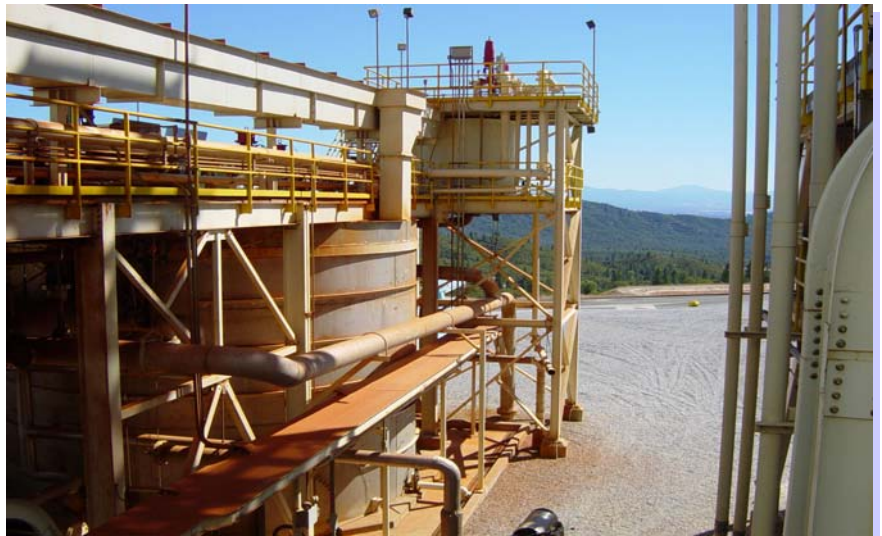
Photo 6: Part of the lime neutralization/high-density sludge acid mine drainage treatment plant at Minnesota Flats. The large tank at center-left is one of two in which acid mine drainage is mixed with lime slurry.
