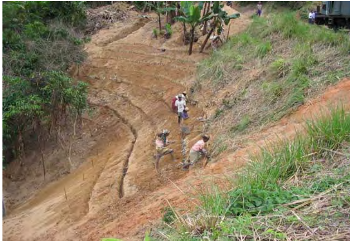
A village based vetiver association was subcontracted by a local engineering firm to plant vetiver to stabilize a drainage infrastructure on the FCE.
