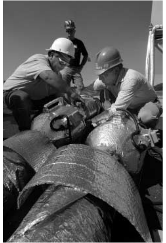
MEMBERS OF KTF'S pad crew disassemble cooling conduit used to keep parts of the rocket at the optimum temperature prior to launch. Clockwise from lower left are Warren Kawaguchi (15419), Jim "Mack" McDonald (Orbital), and Hovey Corbin (15419).
