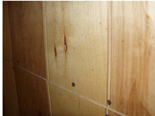
Figure 4-14b. Damage to wood panel following impingement by sparklers from gerb. Lip on panel surface can be seen as line below mounting screws.
