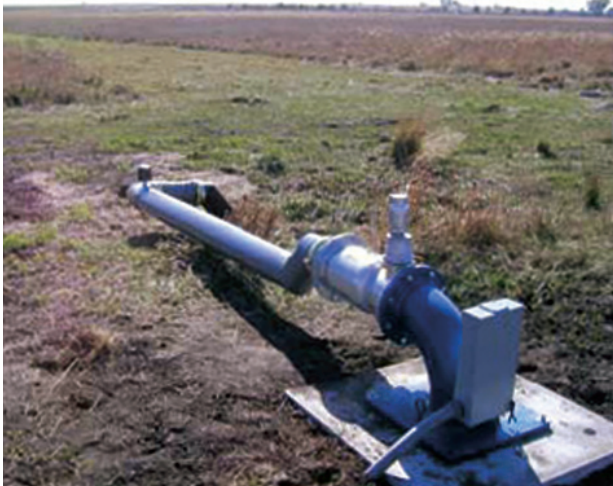
New submersible pump at Harvard WPA (Clay County).
