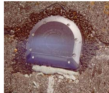
In-Pavement Crosswalk Lighting
