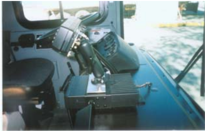
Figure 4-19: ITS Equipment Inside Island Explorer Bus: Voice and Text Communications and Passenger Counter 23
