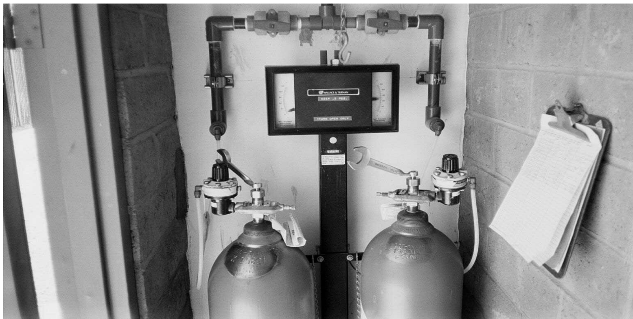
Photo 35. Chlorine System (Subsection 4.3.1.1)
