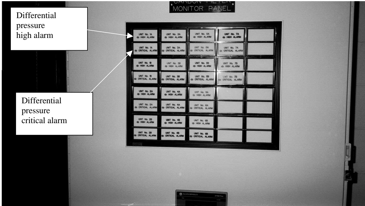
Photo 29. North Plant Alarms (Subsection 4.2.8)
