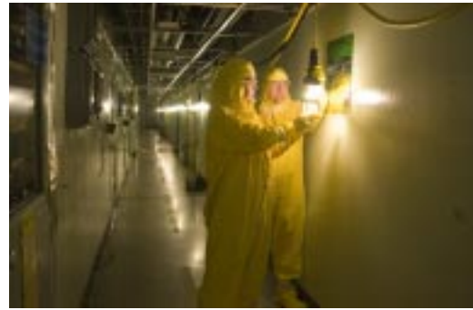
SRS employees hang string lighting in an FB-Line corridor. These lights provide the only illumination in an otherwise pitch-dark facility.
