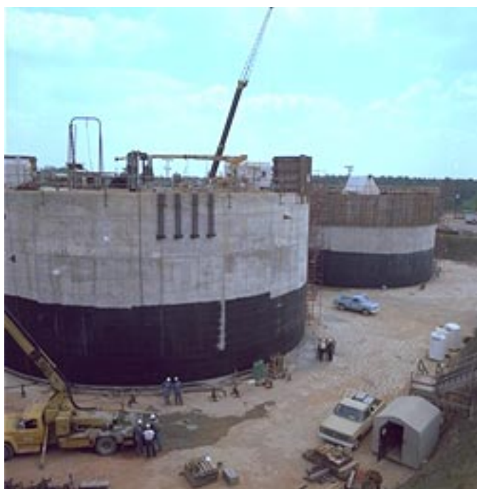
Construction of 51 high level waste tanks began in the early 1950's and continued until 1981.
