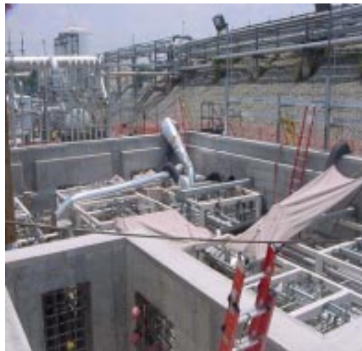
Work on the Modular Caustic Side Extraction Unit (MCU) continues as teams work to modify waste transfer lines. MCU will process waste before it is transferred to Saltstone or the Defense Waste Processing Facility for final disposition.
