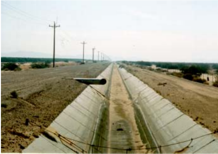
Photograph V-2.—PRPU conveyance system.
