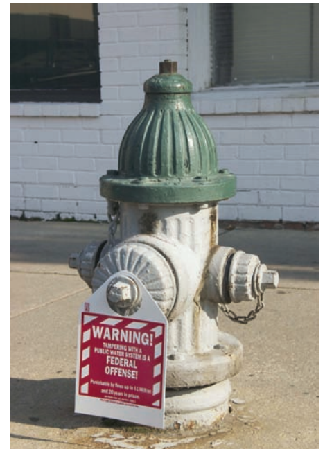
A sign warns against tampering with this hydrant
