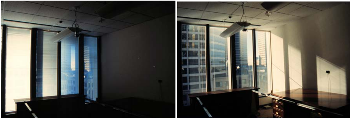
Figure 2 Smart controls on the automated blind systems (left photo) keep direct sun out of the space, reducing glare and cooling loads. The same hardware system with different control strategies (right photo) admits sunlight to offset heating loads but creates excessive glare.
