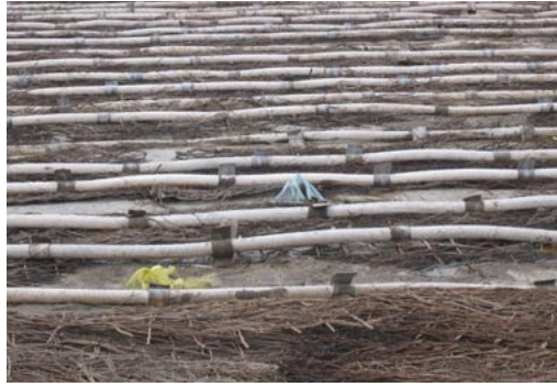
Technology being used to reclaim land in Tianjin by draining pore water from fill material in Bohai Bay.
