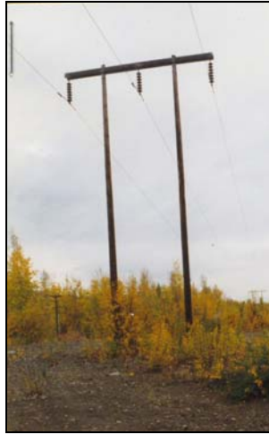
Existing 115 kV Pole
