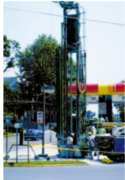
Underground storage tanks that contain gasoline and other fuels can be a source of VOCs in ground water. The drill rig shown above is used to install monitoring wells so the property owner can determine whether leakage or contamination has occurred.
