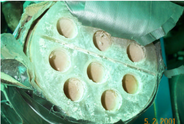
10. Photograph at left shows a closeup of resin column of wastewater treatment plant with yellow dust substance caked within.
