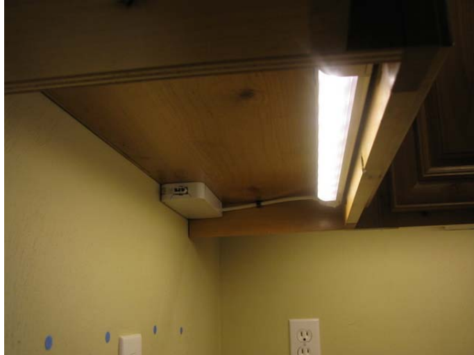
Figure 3.2. Installed LED Undercabinet Fixture
