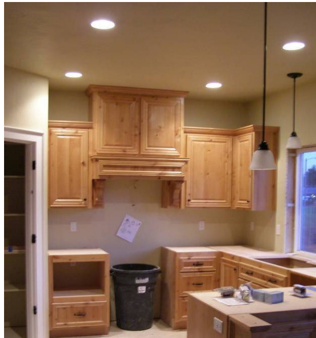
Figure 3.1. Installed LR6 Modules at the Lane County HBA Tour Home
