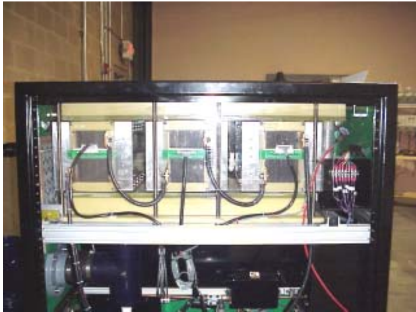
Figure 2-10. Left view of the fuel cell cabinet showing the three fuel cell stacks
