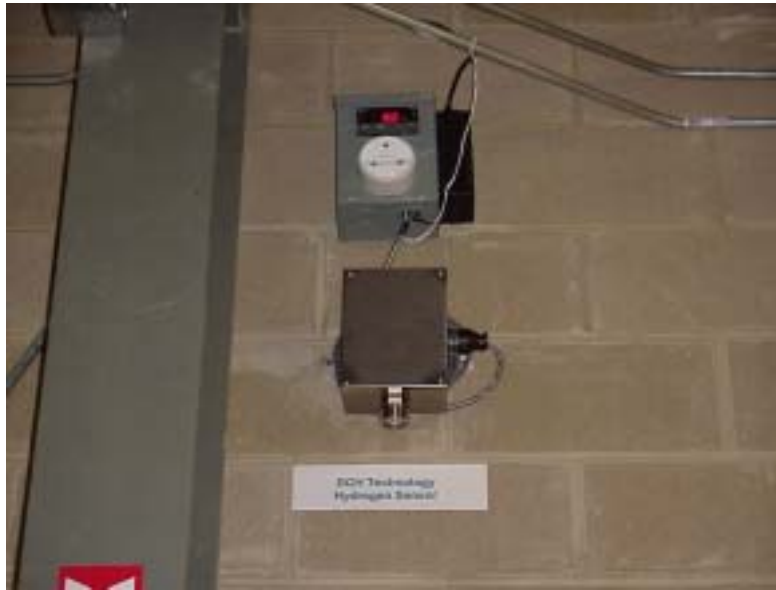
Figure 2-5. The hydrogen sensor mounted near the ceiling above the hydrogen tanks (The sensor was required by local fire code)
