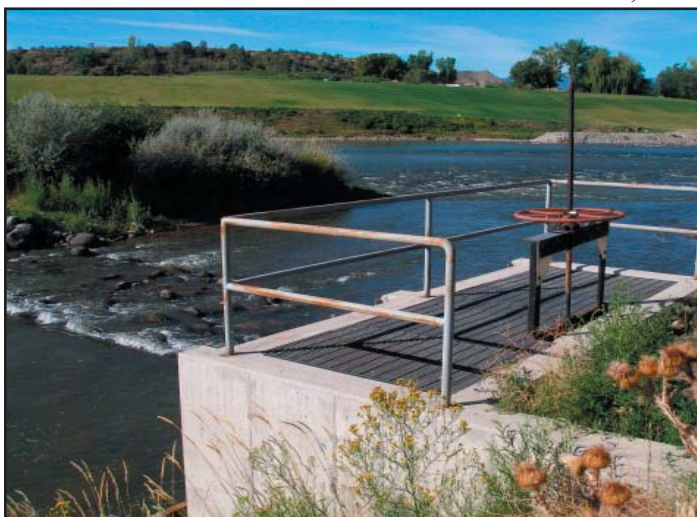
Attendees at the Colorado River Watershed tour were able to view the Silt Diversion Project that was built in 2000 as a means to divert water that will be used in irrigation systems.
