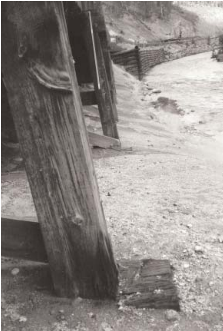
Acidic soils have caused the support piers of the Beryl Spring bridge to deteriorate.
