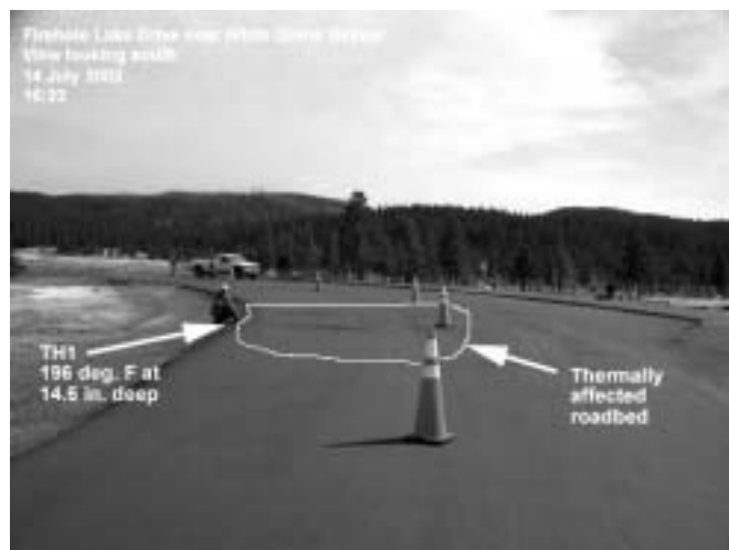
Graphic showing the area of the Firehole Lake Drive damaged by nearby thermal activity.
