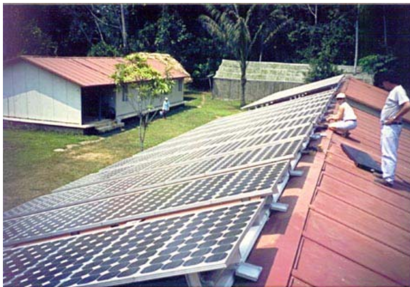
Figure 5. A hybrid photovoltaic-propane generator system now provides facility power for the Chajul Biological Station in the Montes Azules Integrated Biosphere Reserve in Chiapas.
