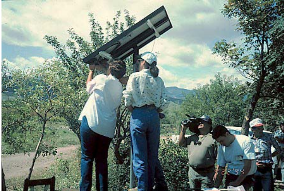
Figure 4. Training activities are tied into the implementation of pilot-projects, such as this photovoltaic water-pumping system installation in Buena Vista for the Chihuahuan Renewable Energy Working Group.
