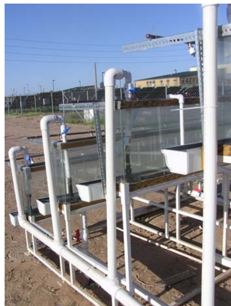
Figure 7. A PVC manifold system conveys compressed air into individual glass tanks for aeration.
