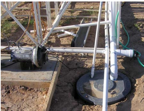
Figure 10. A underground cooling water reservoir receives the water from and delivers to glass tanks using a sump pump.
