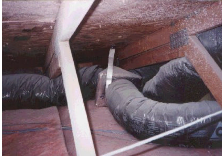
Figure 4. New plastic flexible ducts in an attic
