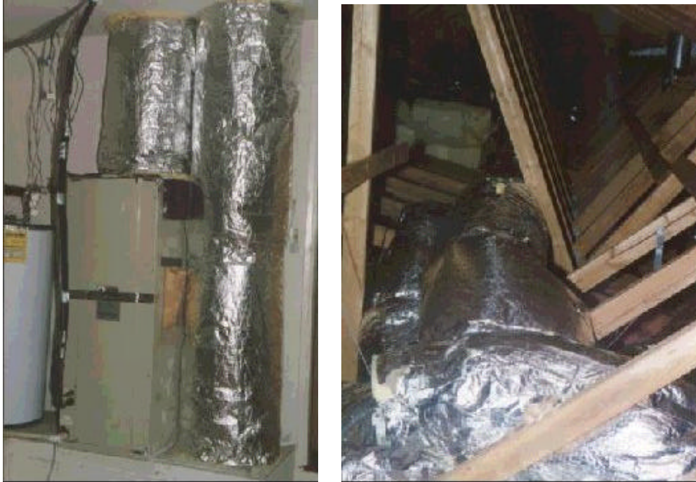
Figure 8. Ducts with added insulation as part of a duct system retrofit.
