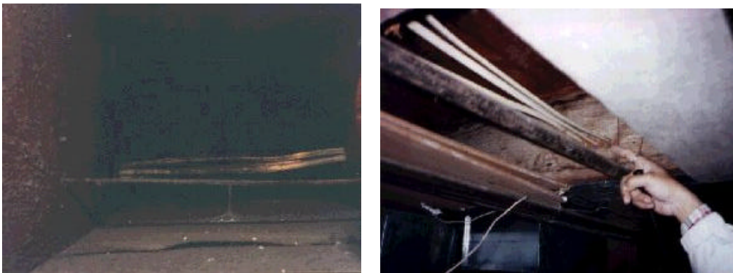
Figure 9. Wires passing through panned joist return ducts
