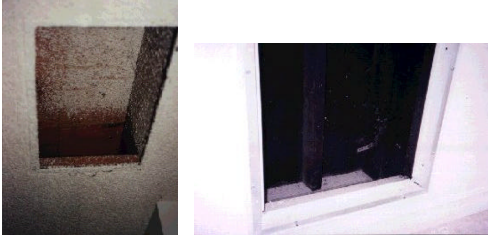
Figure 10. Building cavities used as ducts
