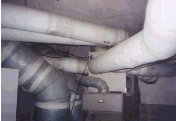
Figure 2. Sheet metal ducts in a basement insulated with asbestos
