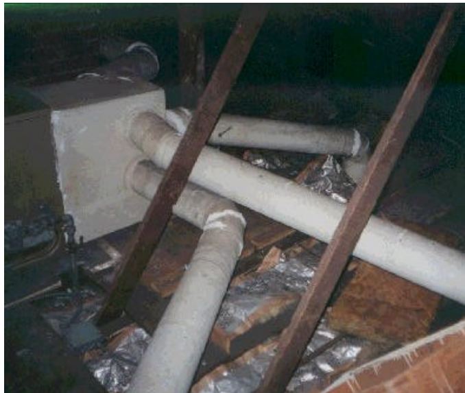
Figure 3. Asbestos insulated sheet metal ducts in an attic
