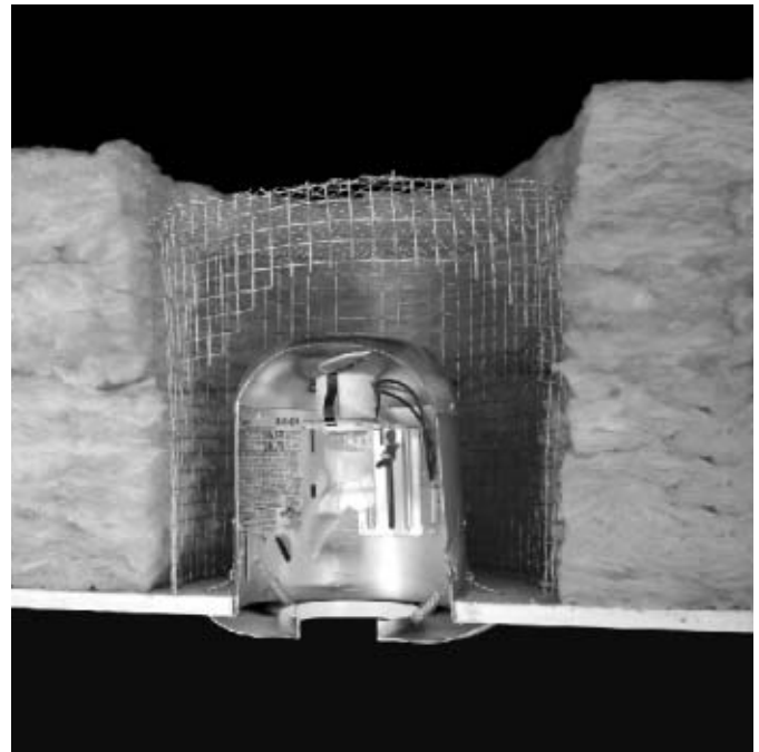
USE SHEET METAL OR WIRE MESH TO HELP CREATE A BARRIER AROUND FIXTURES OR VENTS.
