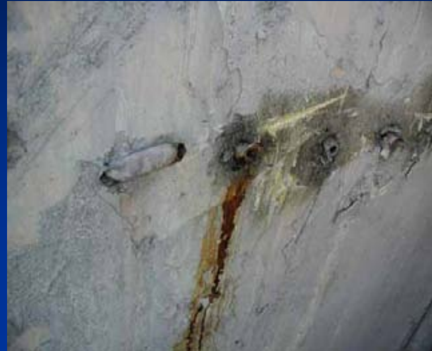
Pipe With Legacy Nitric Acid...Found When Cut
