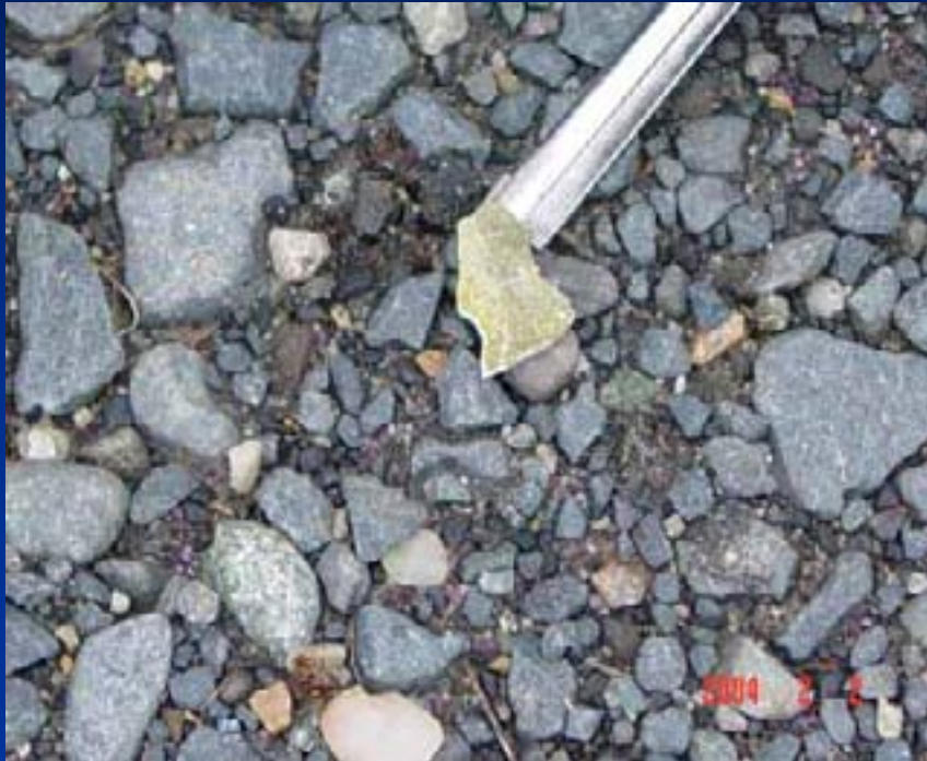
Contaminated Paint Flaking Off Pipes
