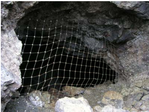
Steel cable netting, State of Texas mine, CNM
