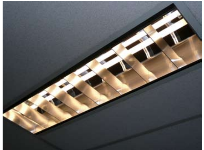
New lighting was installed at Seattle office building (home to most of the Federal Program Team)
