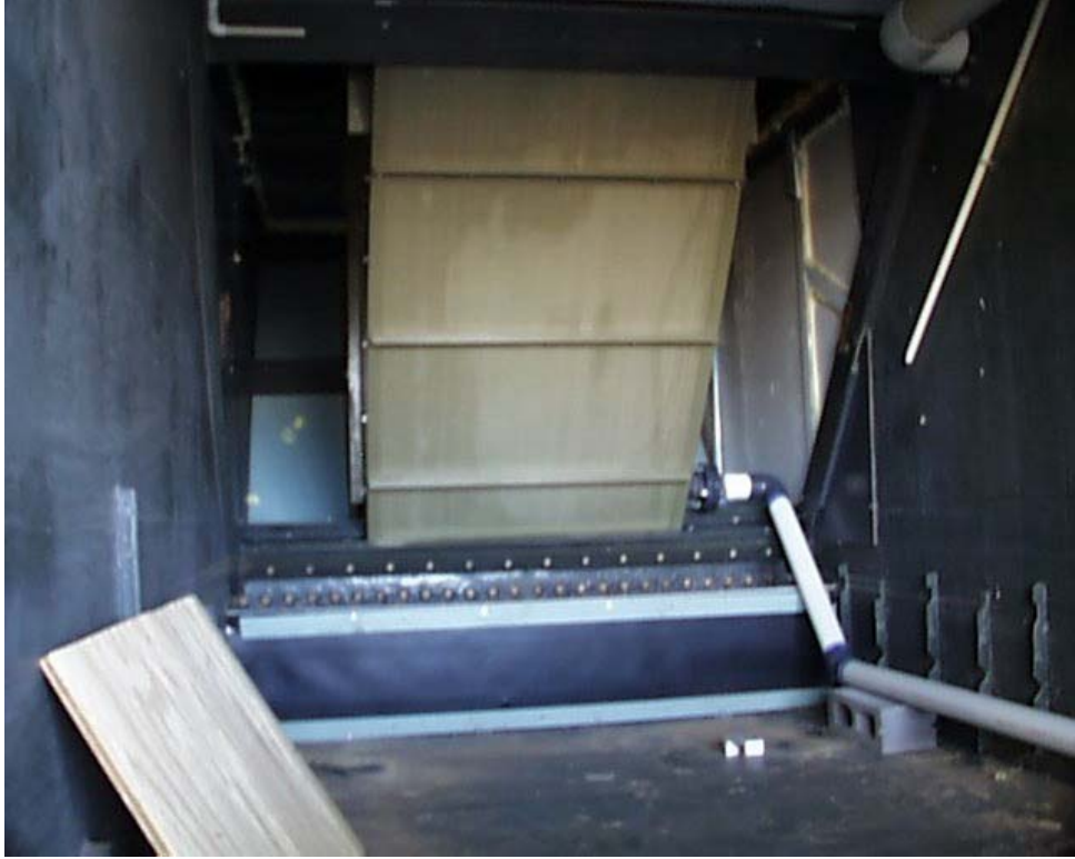
Figure 8.—Basin of the cold evaporation chamber.
