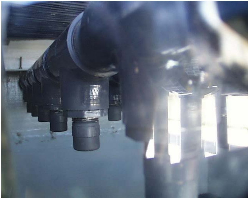
Figure 11.—Spray nozzles at the top of the packed condensation duct.
