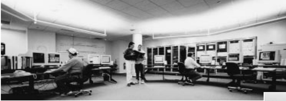
← The APS main control room.
