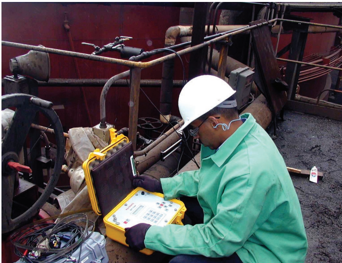
Daryl Cox of ORNL takes a flow reading on a plant pumping system using an ultrasonic flow meter. The ORNL engineer provides technical assistance to help industries identify energy-saving opportunities.
