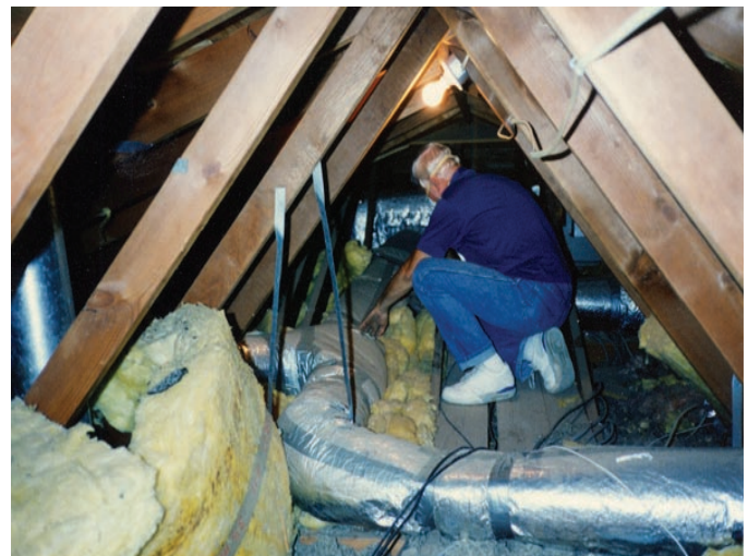
Attic insulation is one of 34 measures that NEAT might recommend to save energy and improve comfort.
