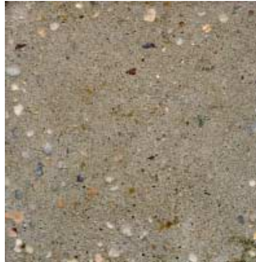
Figure 2. Surface of 10% silica fume concrete after field exposure.
