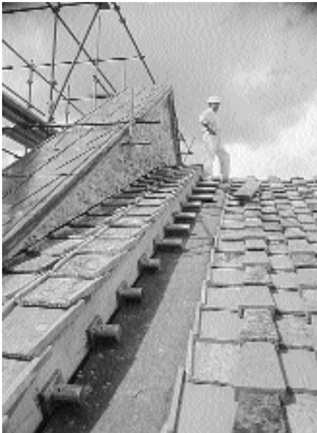
The cylinders that contain the special anchorages connecting the tympanum and the roof.
