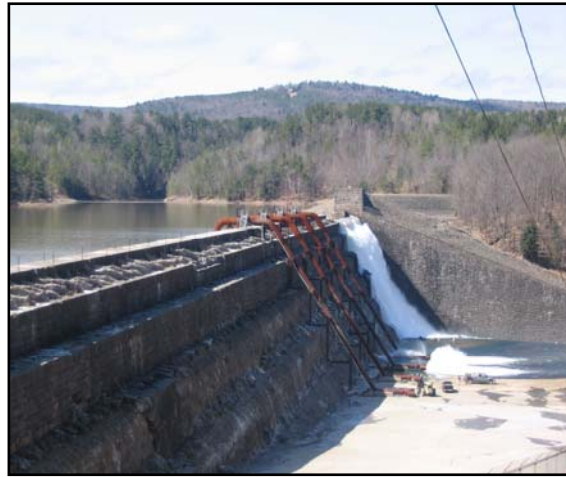
Current Gilboa Dam configuration – lowered principal spillway and 2 siphons working
