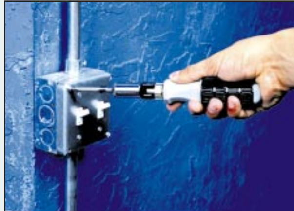
Metal electrical boxes should be grounded to prevent shocks.
