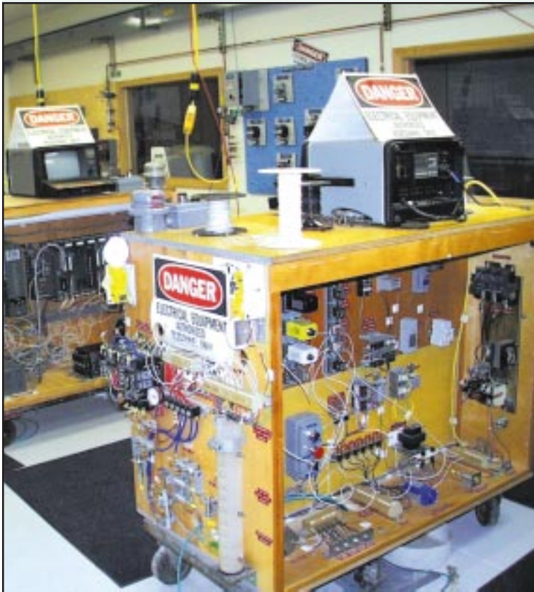
Watch out for exposed electrical wires around electronic equipment.
