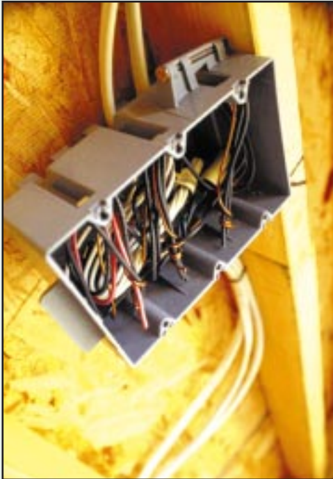
Black and red wires are usually energized, and white wires are usually neutral.
