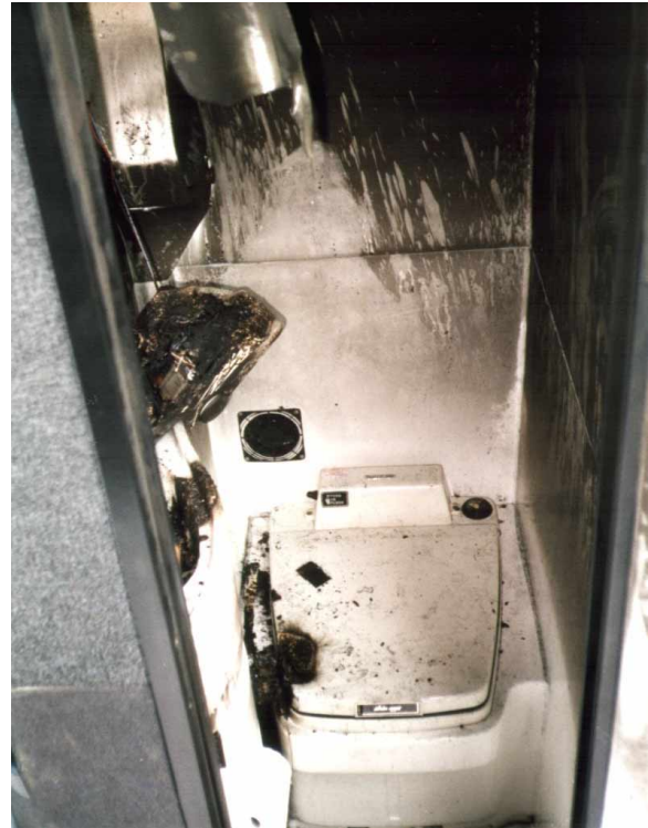
Figure 5 Melted hand-dryer and smoke damage.
