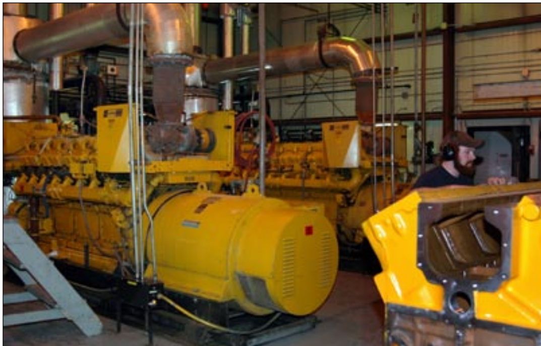
Matt Strine works in front of some of the massive diesel-powered generators that power McMurdo Station. The National Science Foundation plans to install wind turbines in the next few years to reduce the U.S. Antarctic Program's reliance on fossil fuels.
