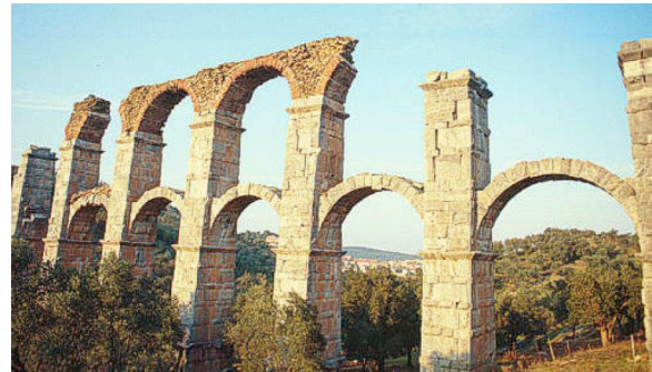
Figure 8. Above ground aqueduct vulnerabilities were exploited by invading threats and suffered from erosion.
