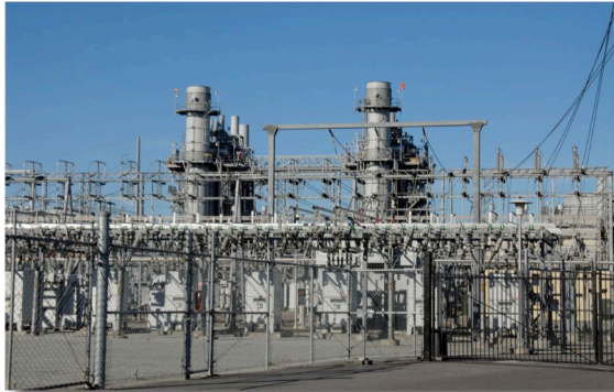
Figure 4. Modern electric infrastructure.
