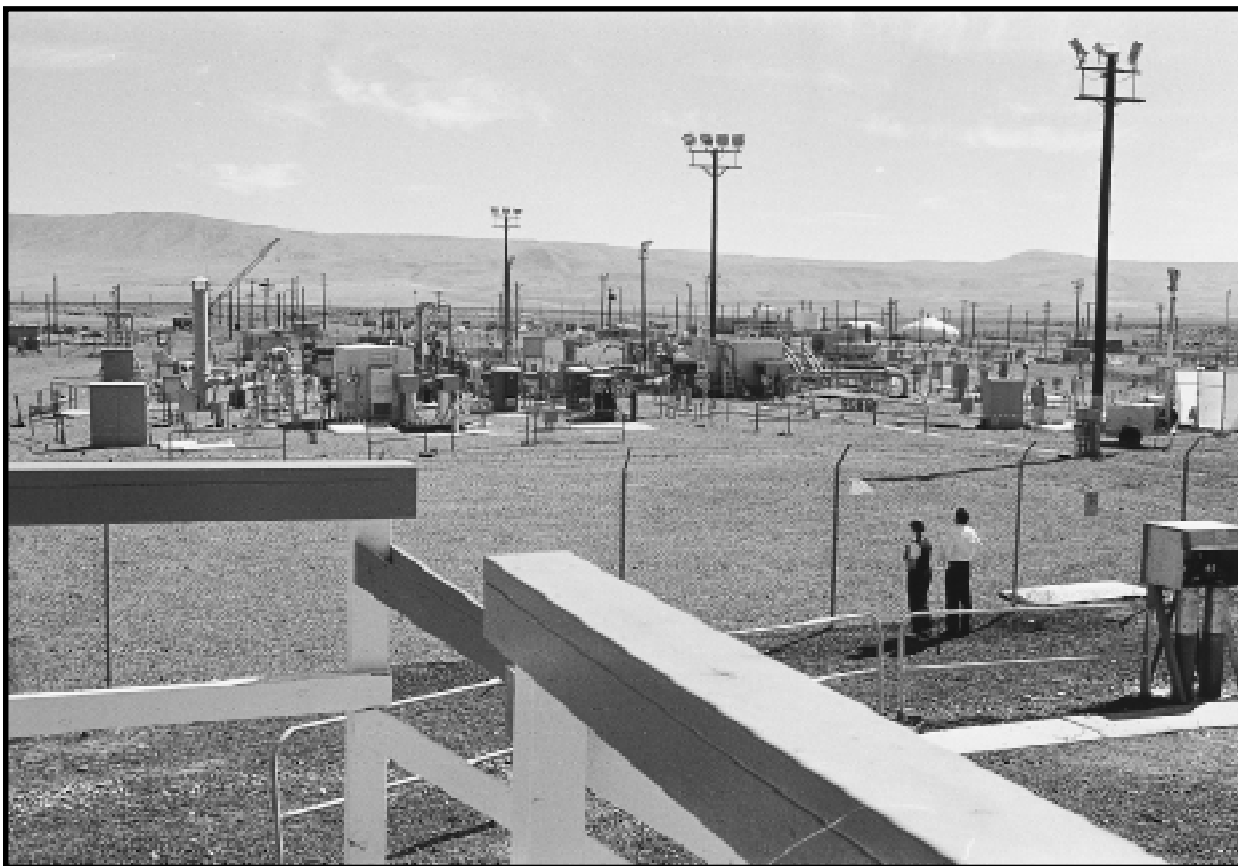
Hanford "Tank Farm." The million-gallon double-walled carbon steel tanks buried here hold high-level nuclear waste from Hanford's plutonium production program. The double-walled tanks have replaced Hanford's older, single-walled tanks which have leaked approximately one million gallons of high-level radioactive waste into Hanford soil. 200 Area, Hanford Site, Washington. July 12, 1994.
