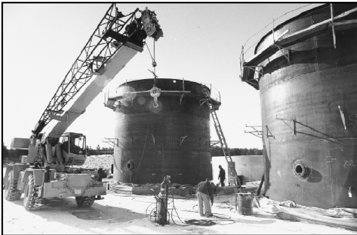
Advanced waste water treatment facility under construction. Fernald Environmental Management Project, Ohio. December 28, 1993.
