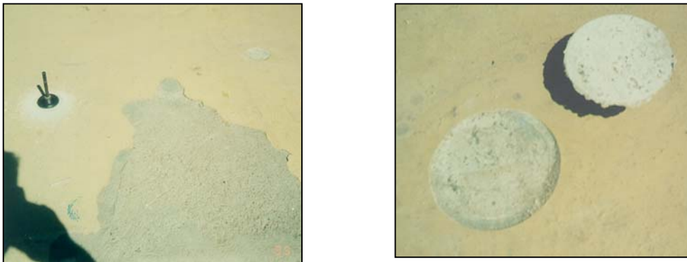
Figure 20. Example of deteriorated industrial floor and evaluation of adhesion with pull-off test
