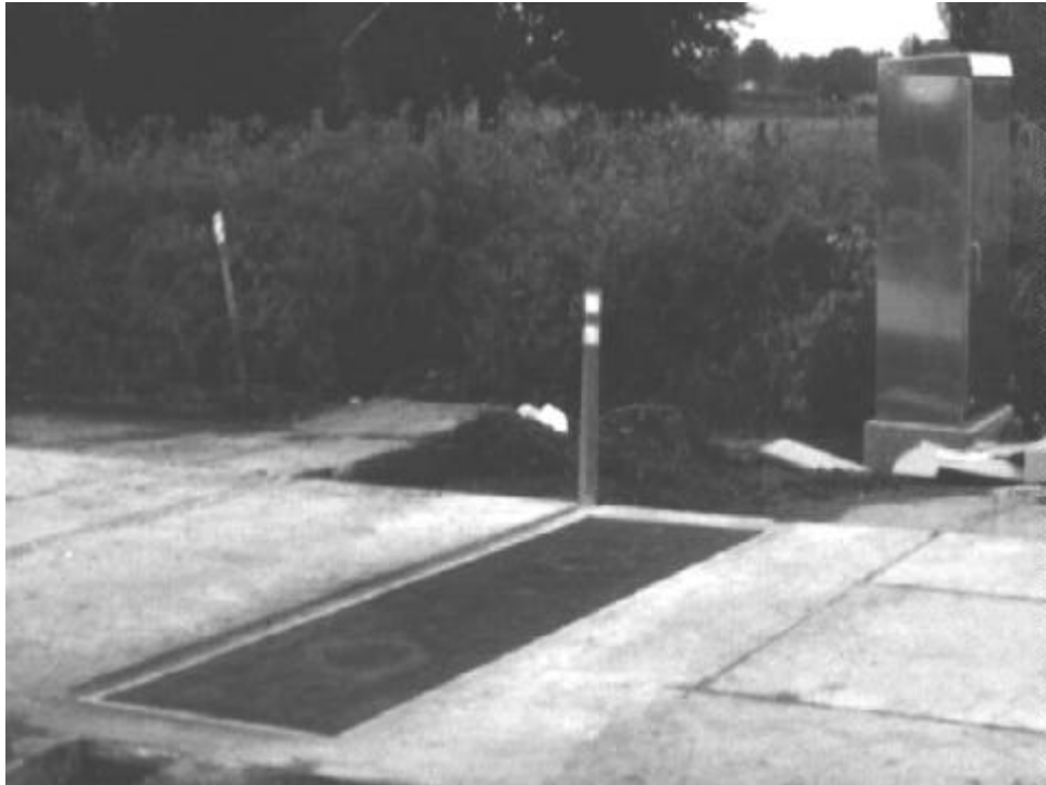
Figure 5.4 Installed Load Cell Scale
