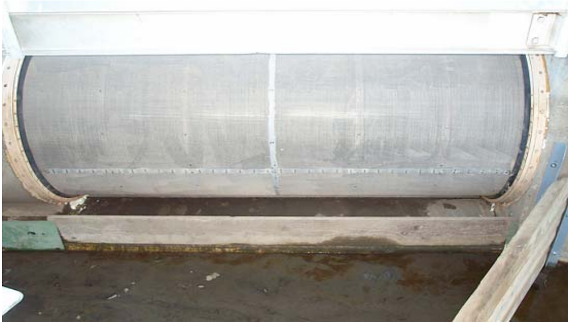
Figure 26. Screen 1 at Naches-Cowiche with Stoplogs in Front of the Screen (parallel) and Upstream of the Screen Bays (perpendicular to the direction of water flow). The upstream stoplogs were blown out by high flows early in the irrigation season.
