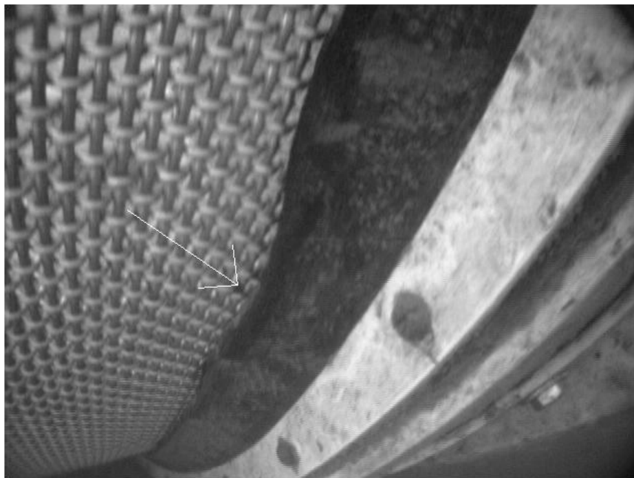
Figure 30. Damaged Seal at New Cascade, Downstream on Screen 8
