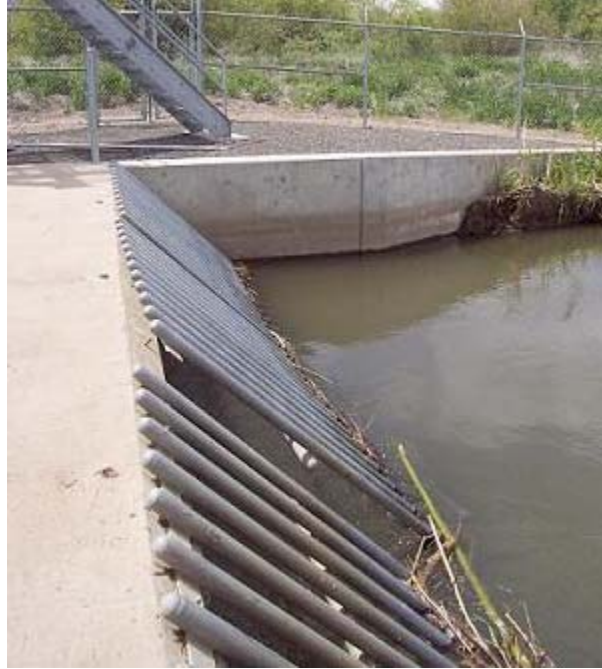
Figure 43. The Trashrack at Toppenish Pump was Partially Separated from the Concrete Wall in May 2002
