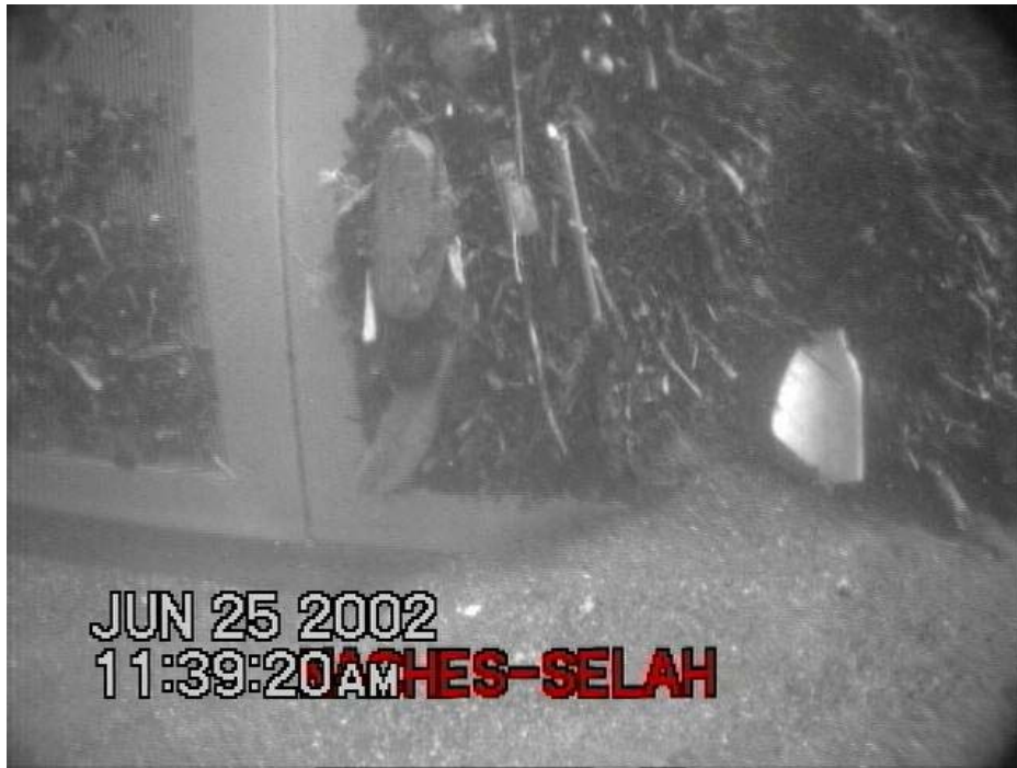
Figure 62. Sediment Accumulation and Debris on Screen 6 at Naches-Selah in June 2002
