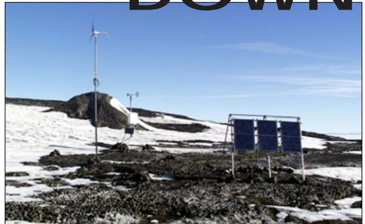
Two wind generators and a solar panel array charge batteries near Arrival Heights. Photo by Kristan Hutchison Sabbatini.
