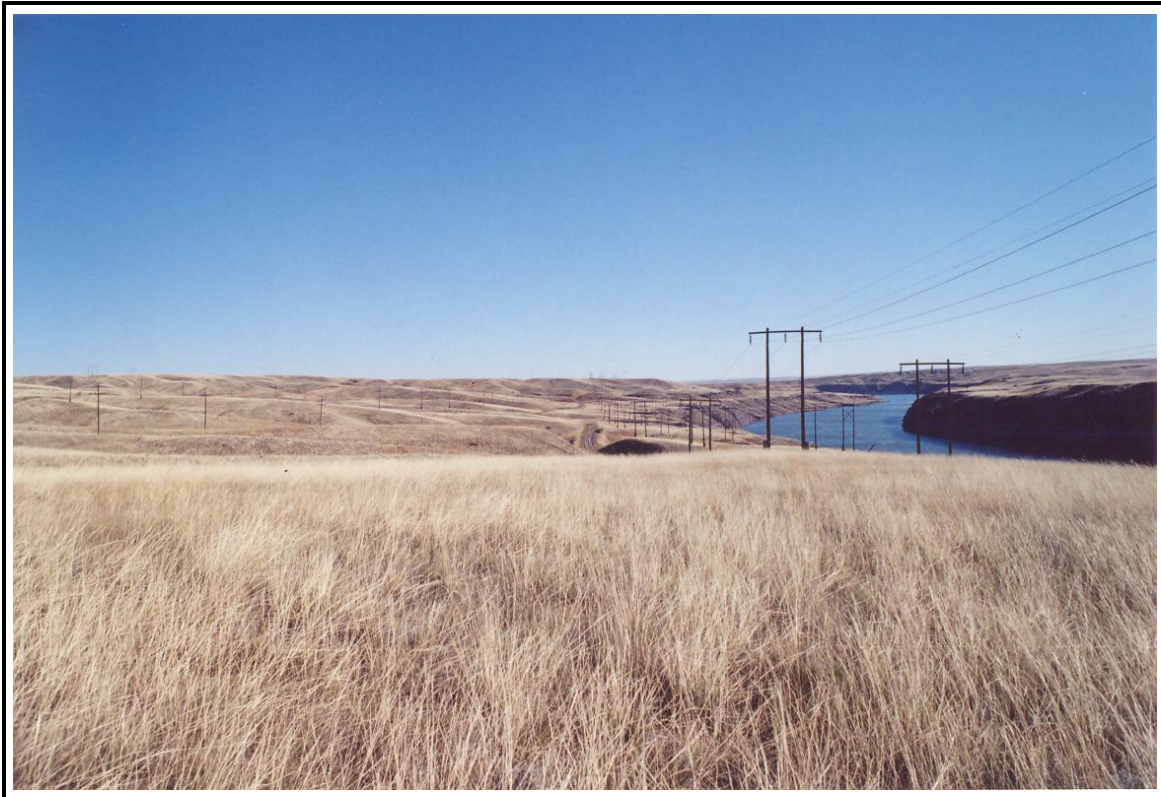
Figure 8. The Morony (24CA289 Feature 2) and Rainbow (24CA291 Feature 34) transmission lines. View to the northeast.
