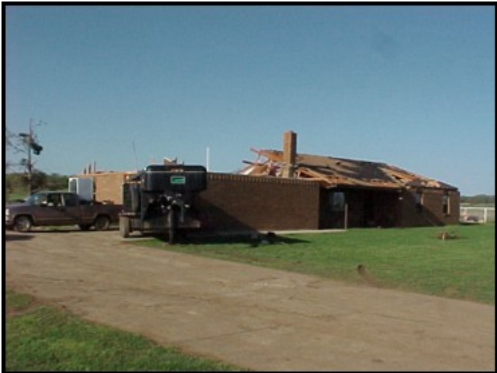
Picture 10: Damage to frame home. Approximately half of the roof has been destroyed with minor damage to most of the exterior walls. Picture is looking northeast. (See Figure 6 for location of picture).
