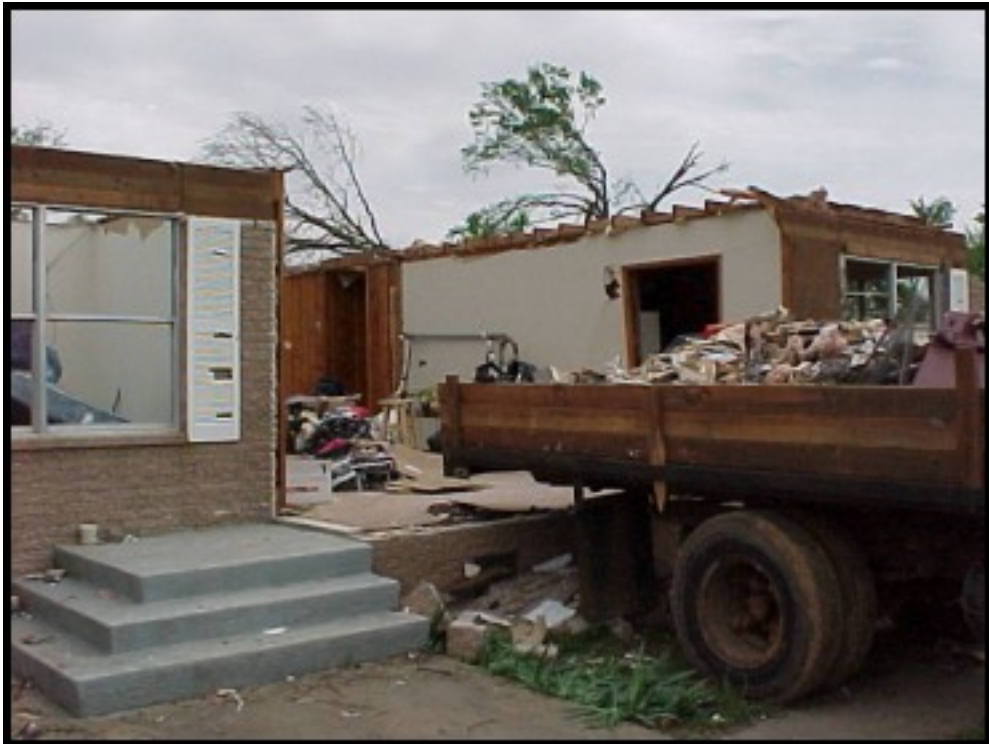
Picture 4: Looking northeast. A frame home was severely damaged 1 mile east of Milburn. The roof was completely removed, and portions of the front and rear walls of the structure were blown out. (See Figure 5 for location of picture).
