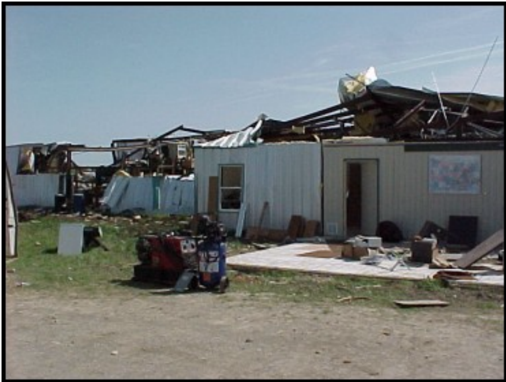
Picture 6: Looking northeast. Severely damaged business 2.5 miles south of Wapanucka. (See Figure 5 for location of picture).
