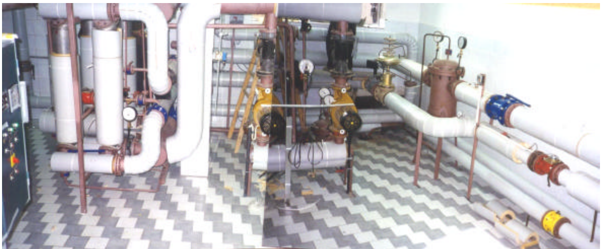
A section of a typical boiler room after renovation and conversion with EAPS assistance, 1997.
