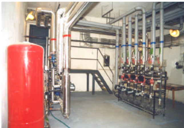
New hot water distribution center in an apartment complex in Vratimov, Czech Republic, 1997. EAPS helped operationalize a joint venture between the town of Vratimov and the nearby Nova Hut steel mill, under which Nova Hut utilized its waste heat (supplemented by heat from a cogeneration facility) for district heating serving 32 percent of the city. This enabled Vratimov to shut down 16 heavily polluting coal-fired district heating boilers.
