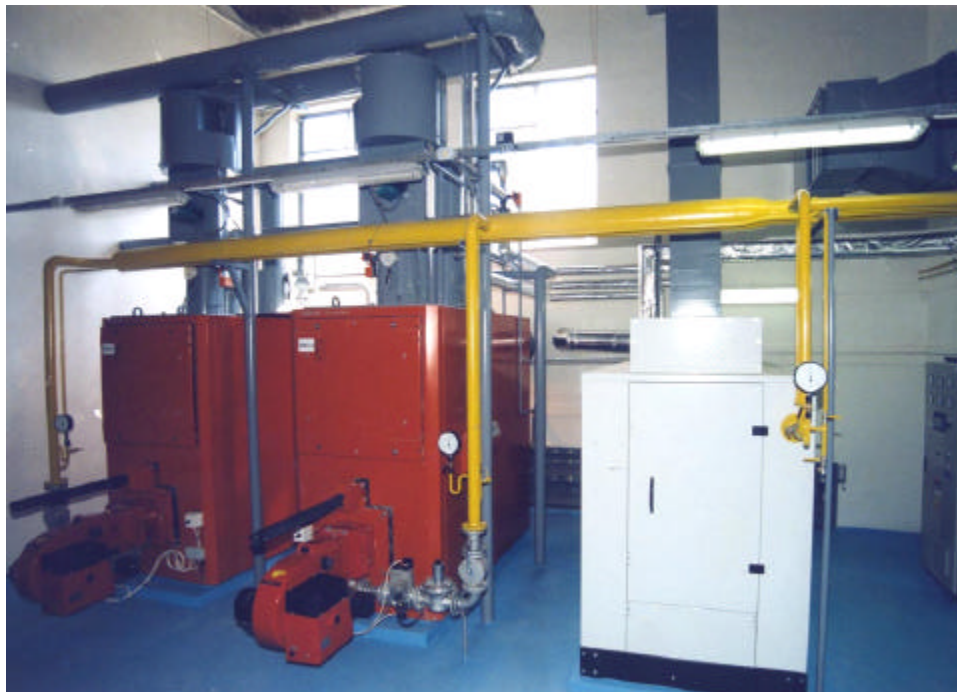
Apartment block furnace room in Krakow, 1997. The EAPS program helped obtain financing to replace heavily polluting, antiquated, coal-fired furnaces with these clean, automated, gas-fired furnaces, including renovating the space to accommodate modern equipment.
