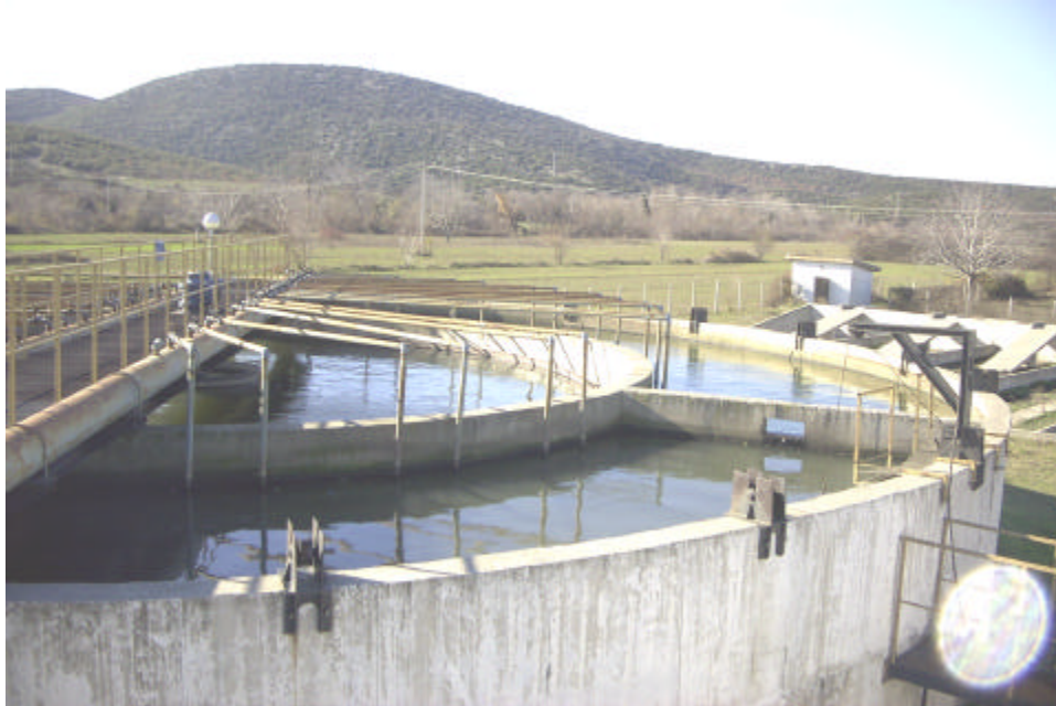
Reactor number 1 before reconstruction at the Dojran wastewater treatment plant, rehabilitated through the EAPS Macedonia program, 2000.
