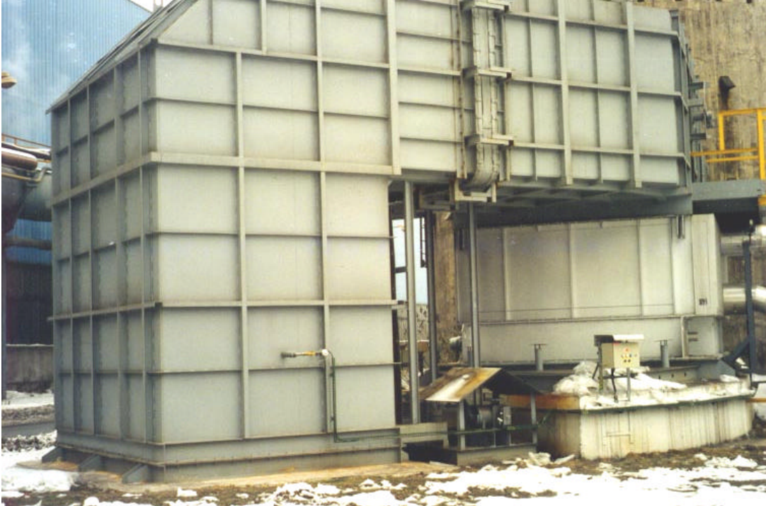
Heat exchanger for utilizing waste heat from the Nova Hut steel mill for district heating in the town of Vratimov, 1997. The EAPS Czech Republic program helped implement this P2 project, which reduced emissions of particulates in Vratimov by 55 percent, reduced sulfur dioxide emissions by 72 percent, and reduced carbon monoxide and carbon dioxide emissions by 93 percent.
