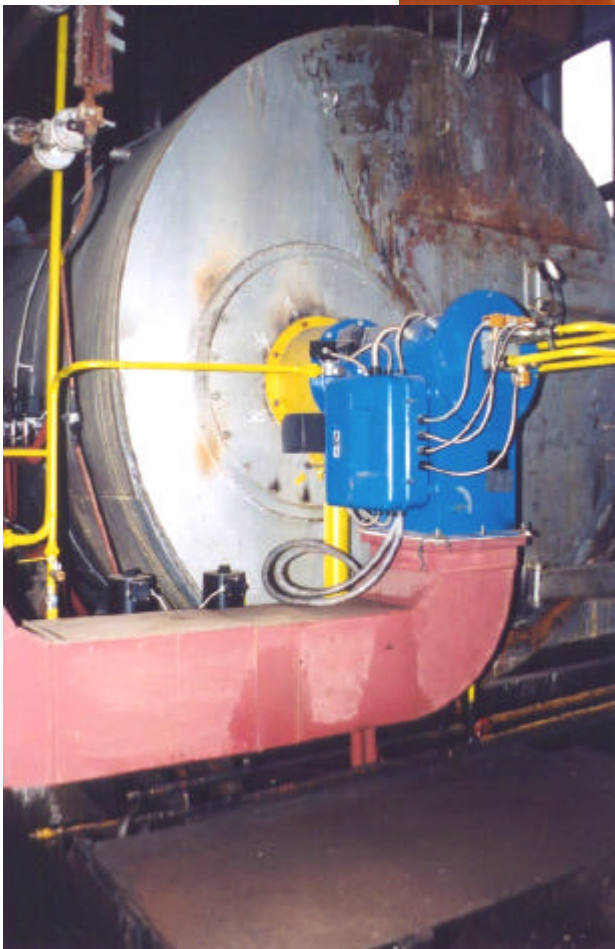
Boiler in Stara Zagora regional hospital, converted from light diesel to natural gas under the EAPS Bulgaria program, 1998. Yellow pipes mean gas.
