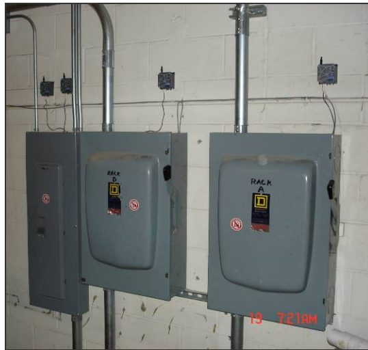
Figure 14. Motes connected to current transducers monitoring energy loads in building sub panels.
