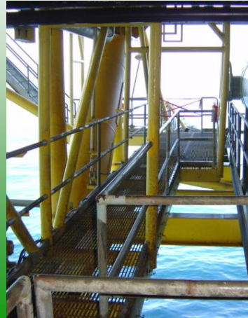
Sub-Cellar deck NW walkway minor lateral displacement
