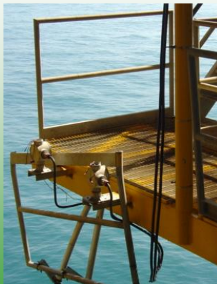
Sub-Cellar handrail damage
