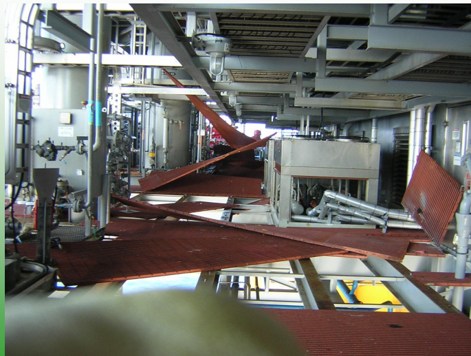
Damage NE Mooring Porch – Debris
