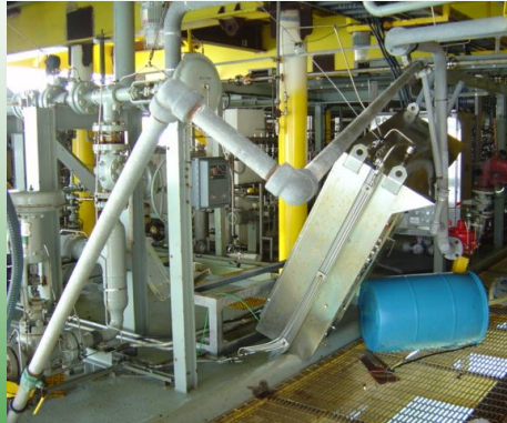
Sub-Cellar typical panel and ancillary piping damage
