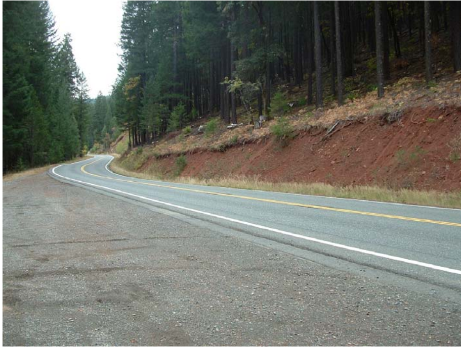
Figure 26. Cutbank on Rush Creek Road.
