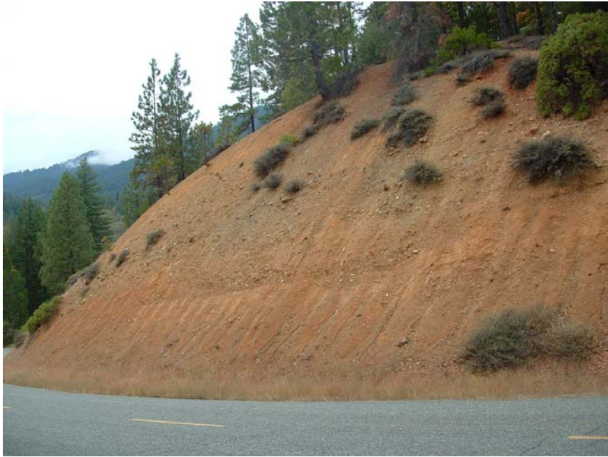
Figure 27. Cutbank on Trinity Dam Boulevard, which exhibits rilling as well as dry ravel.
