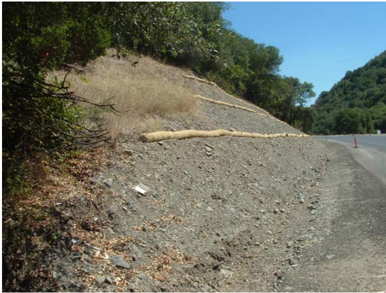
Figure 30. Wattles installed along the contour of a cutbank to trap fine sediment before it enters inboard ditch.
