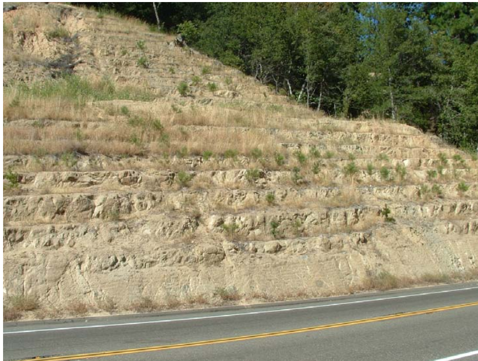
Figure 31. Benches constructed on a cutbank to decrease surface erosion and to encourage revegetation.
