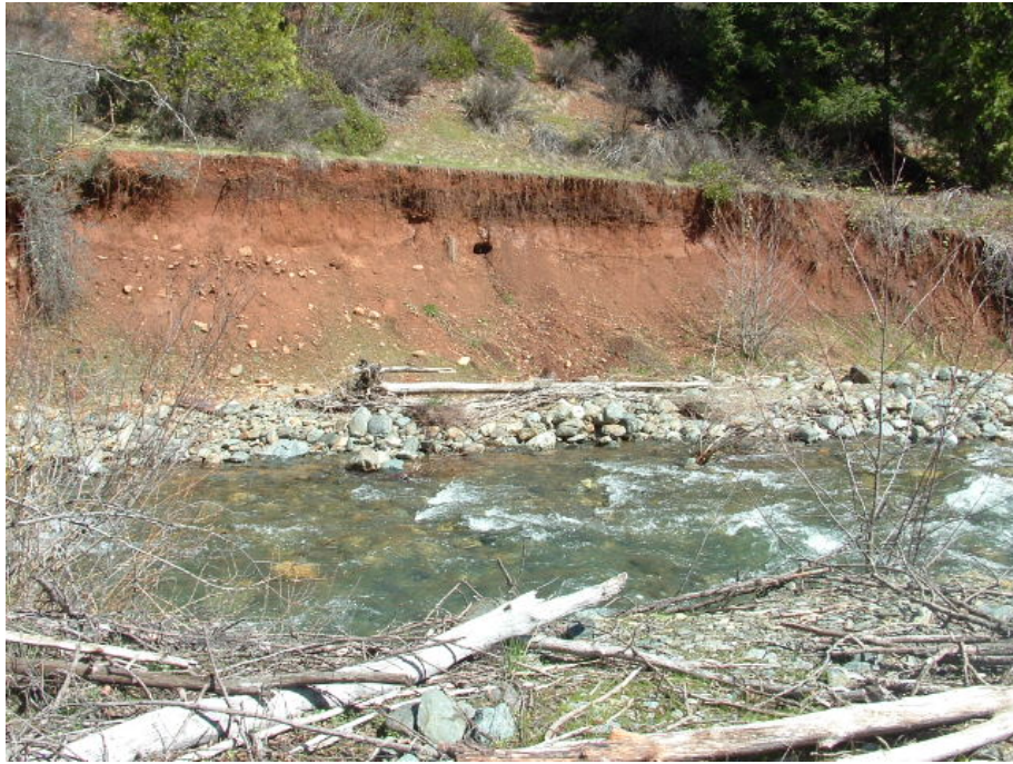
Figure 36. Eroding left bank of Rush Creek upstream of Highway 3.
