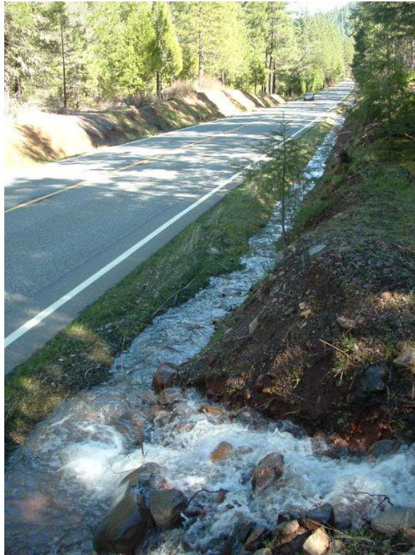
Figure 29. Runoff entering an inboard ditch, which then delivers the water and sediment through a culvert to a perennial stream.
