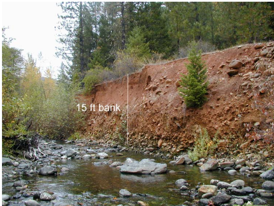
Figure 34. Near-vertical streambank actively contributing sediment to Rush Creek.
