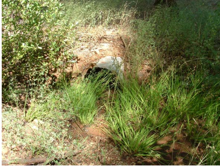
Figure 23. Culverts plugged with sediment are a common problem on forest roads.
