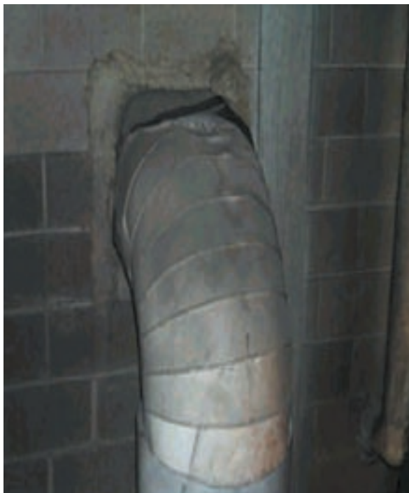
Photo 3a. Partially damaged insulation on a pipe elbow.
