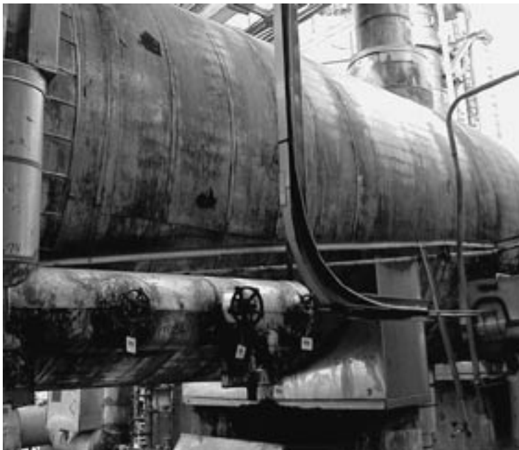
Photo 7. Midwest chemical plant with damaged vapor retarder.
