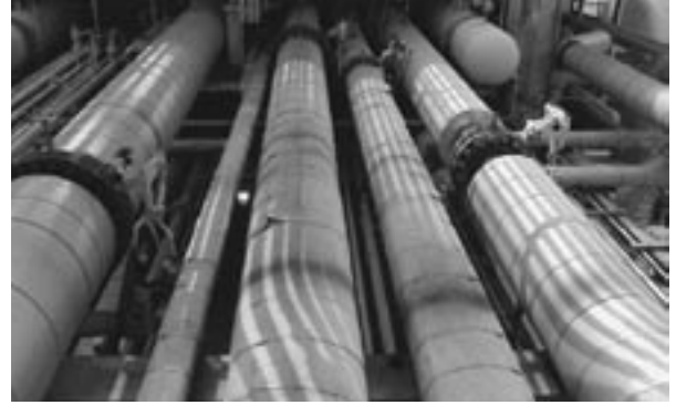
Photo 2. Cosmetic damage on pipes.
