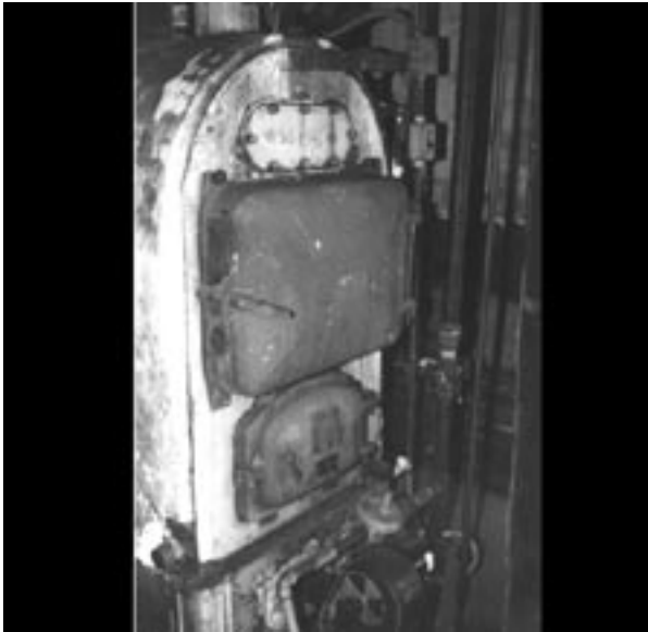
Photo 2. During most inspections archaic equipment like this 60-year-old boiler does not typically get screened for safety upgrades to firing controls.
