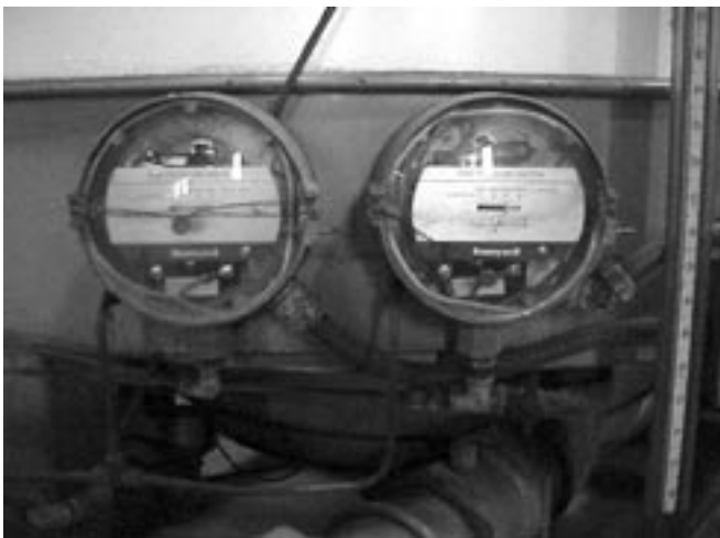
Photo 5. Typical high/low gas pressure switches to verify gas pressures are in the proper range.
