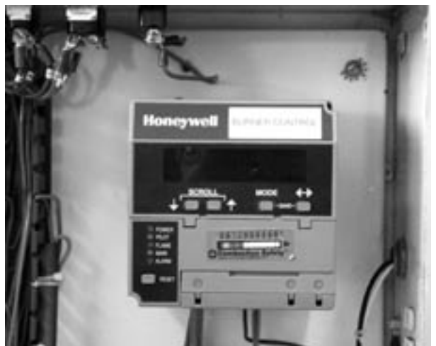
Photo 8. The burner management system is the brain that monitors/directs safe firing and operations.
