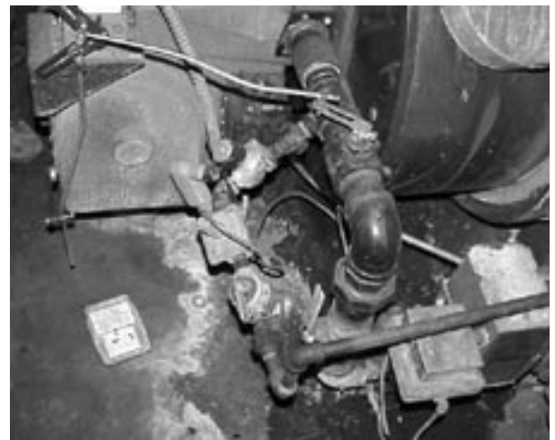
Photo 1. This equipment, in this condition, has been approved to operate “as is” by current jurisdictional inspection practices.
